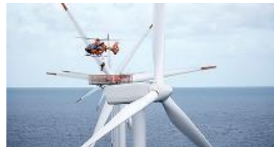
Preventive maintenance of wind turbines
